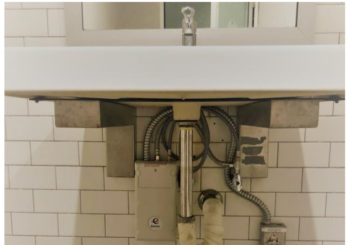
Lavatory Point of Use Heater with instrumentation
