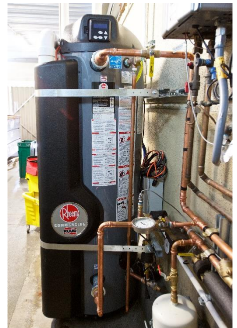
Condensing Storage Heater as Installed Onsite
