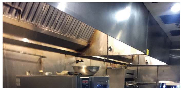
Demand Control Kitchen Ventilation (DCKV) installed in main line hoods
